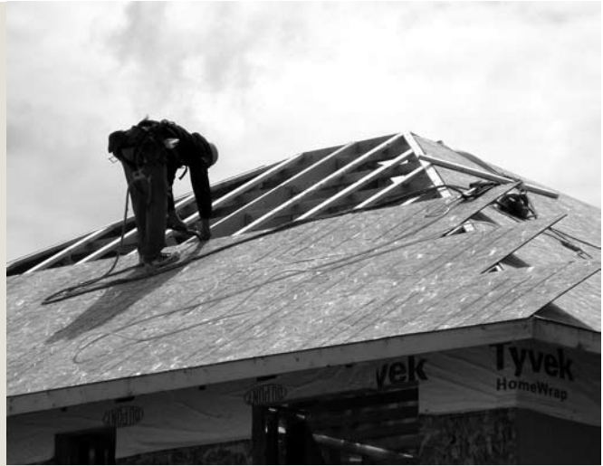
In this fall arrest system, the roof strap is looped and choked around a 2 x 6 inch truss brace.
